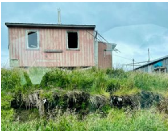
Image 8: Threatened Home Hooper Bay, September 7, 2023
