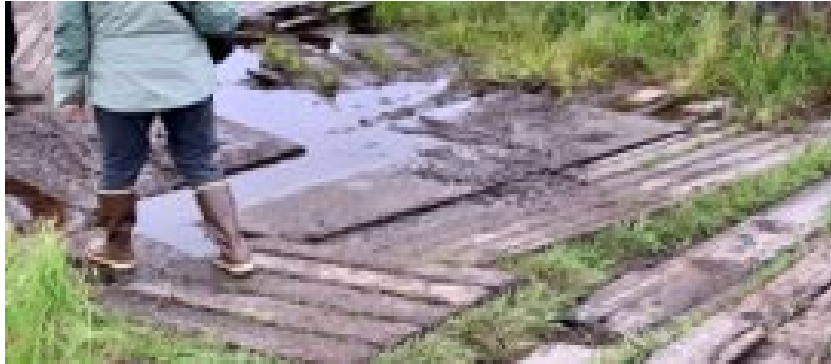
Image 18: Accelerated Permafrost Degradation Tuntutuliak, August 17, 2023
