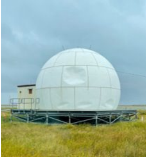
Image 7: Geodesic Home in Hooper Bay Dented by Floating Driftwood and Logs Propelled by Merbok Winds and Storm Surge Flooding that Exceeded 20 Feet in Height, September 7, 2023
